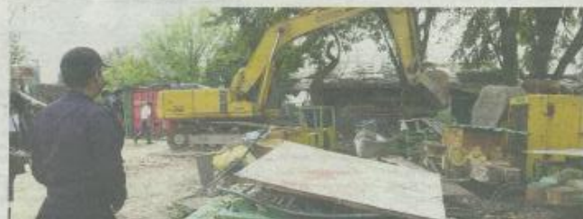
Authorities from MPS and Gombak Land and District Office demolishing a heavy machinery workshop that was built illegally along the river banks of Sungai Garing, Rawang, on Dec 1
