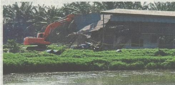
Structures at the fish farm in Hulu Selangor being demolished. – Photo courtesy of LUAS
